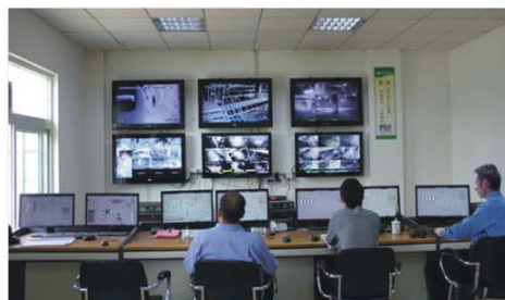
Master control room
